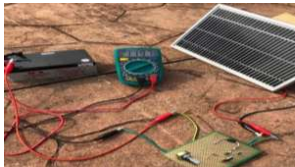
Figure 5 Solar PV cell with the charge controller and battery
